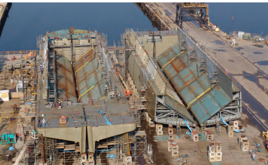
Two dump scows for Great Lakes Dredge & Dock Company under construction in Mobile.
